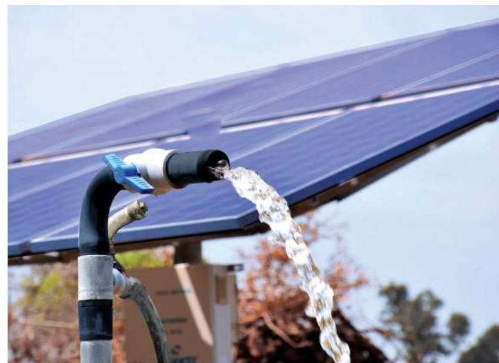
Solar Powered Water Pumps
